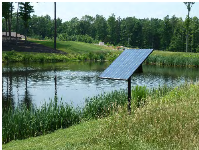
Figure 33. Solar energy powered pond aerator at the Federal Club.
