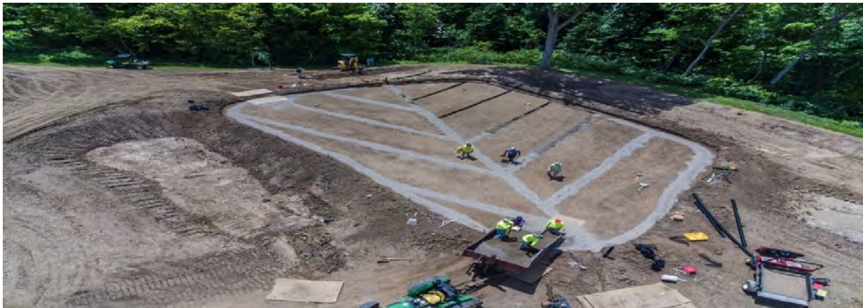
Figure 3. When constructing drainage systems, pay close attention to engineering details such as subsoil preparation, the placement of gravel, slopes, and backfilling. Photo credit: Jason Mahl.
