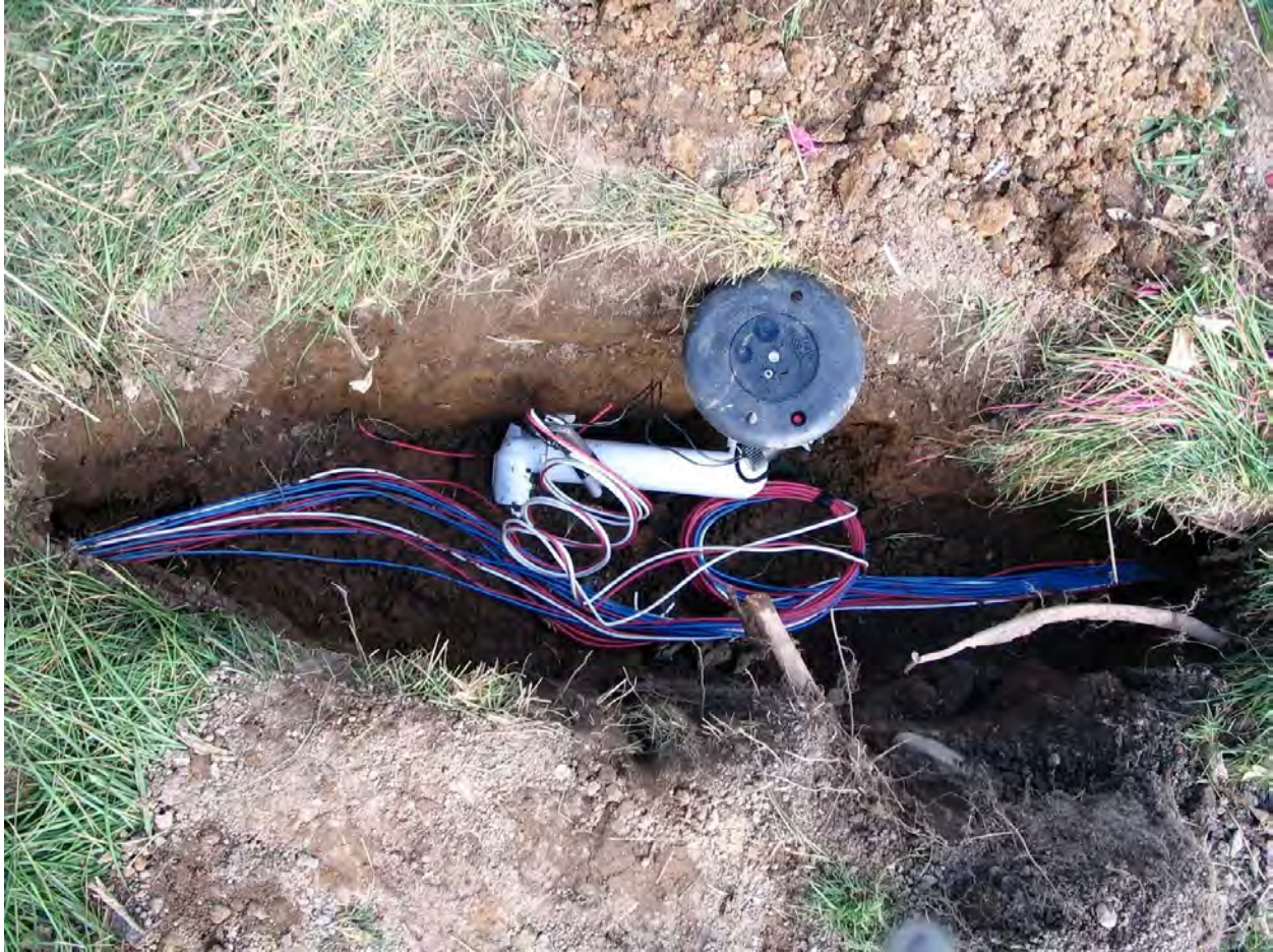
Figure 8. System checks and routine maintenance on pumps, valves, programs, fittings, and sprinklers should follow the manufacturer's recommendations. Photo credit: Jason Mahl.
