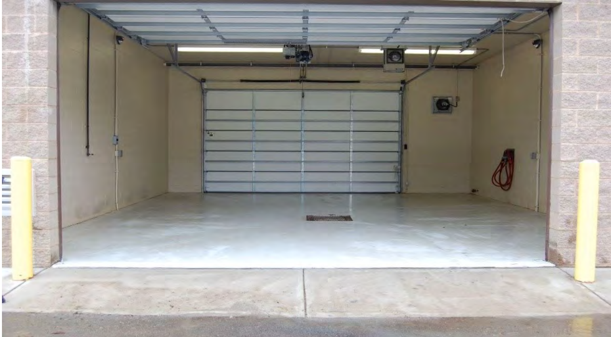
Figure 4. Construct floors of seamless metal or concrete sealed with a chemical-resistant paint. Photo credit: Jason Mahl.
