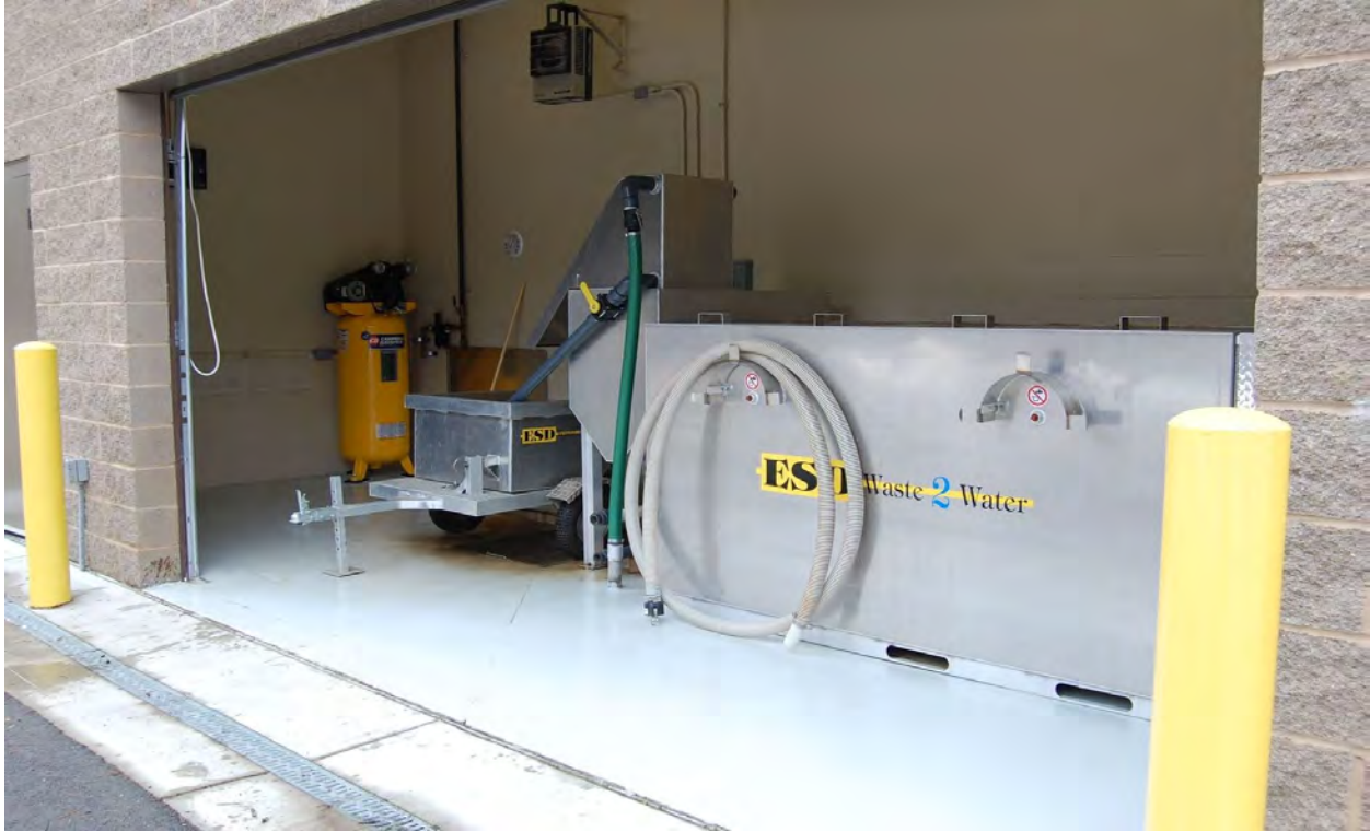
Figure 33. Wash equipment over a concrete or asphalt pad that allows the water to be collected. Photo credit: Jason Mahl.
