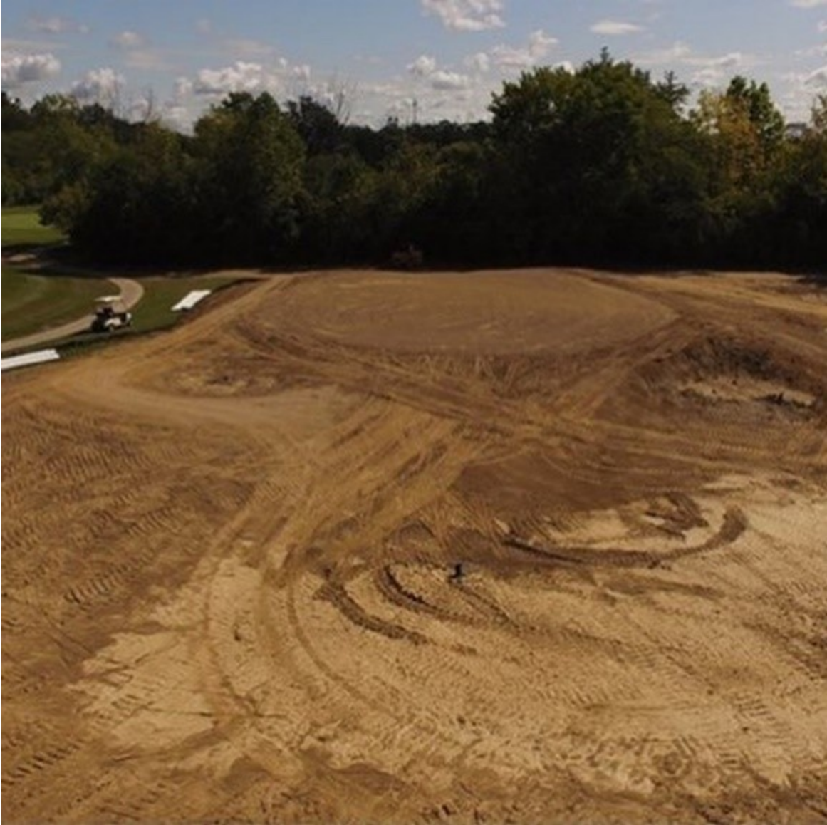
Figure 2. Construction and shaping of a green complex at Cross Creek Golf Club, Decatur, IN. Photos courtesy of Brandon Razo.
