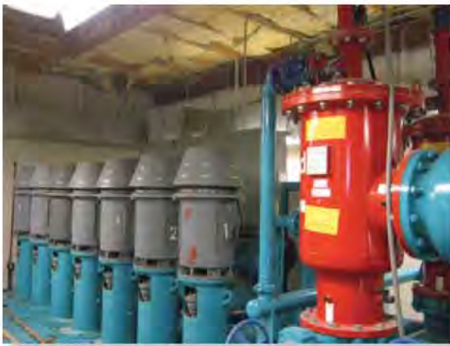
The pump station for the Chiricahua Course, The Desert Mountain Club, Scottsdale, Ariz. The golf course has saved on its energy costs by reducing the total number of horsepower used to pump water. Photo by Jim Key, CGCS
