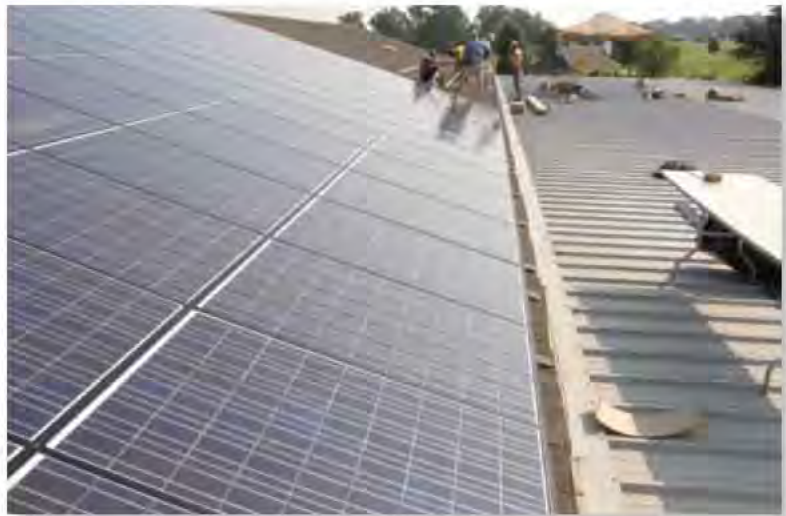
Installing a solar power operating system is expected to significantly lower the electric bill at the Island CC in Plaquemine, La. Photo by David McCallum
