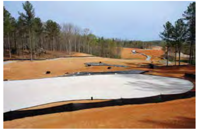
Figure 2-9. Using a variety of materials to avoid soil erosion during on a golf course construction site.
