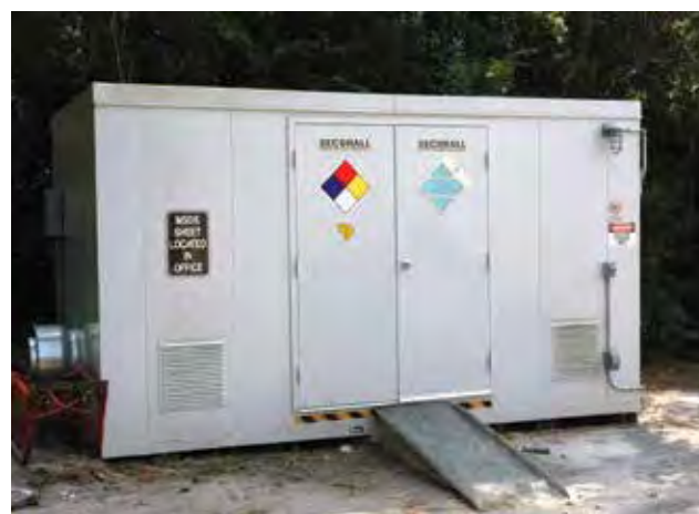
Figure 11-6. A prefabricated pesticide storage facility.
