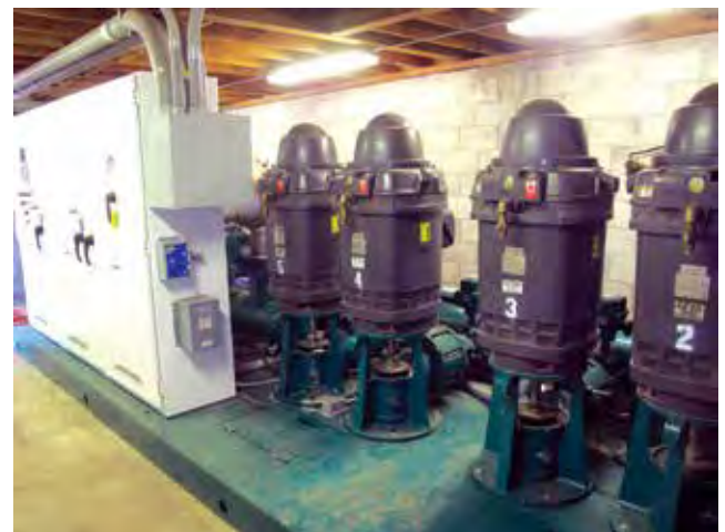
Figure 3-12. A typical computerized irrigation system using the most energy efficient variable frequency drive pumps.
